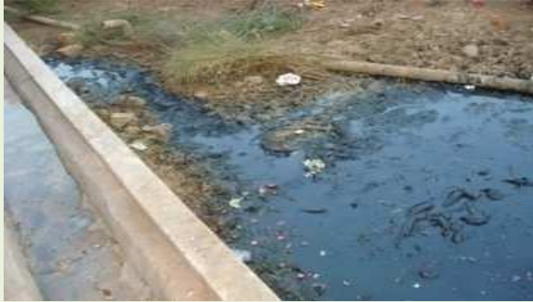
Open drainage in Integrated Hostel Welfare Complex Nandyal, Kurnool district
