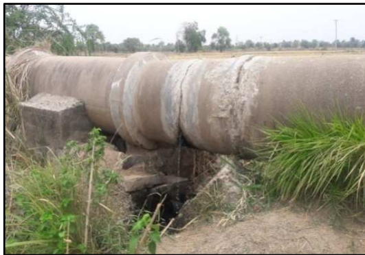
Bodhan ULB (Leakage from pipeline)
