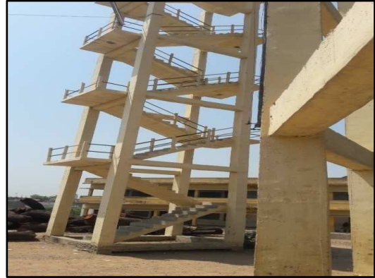
Non-provision of railings to stair case of 1 st and 2 nd flights of ELSR
